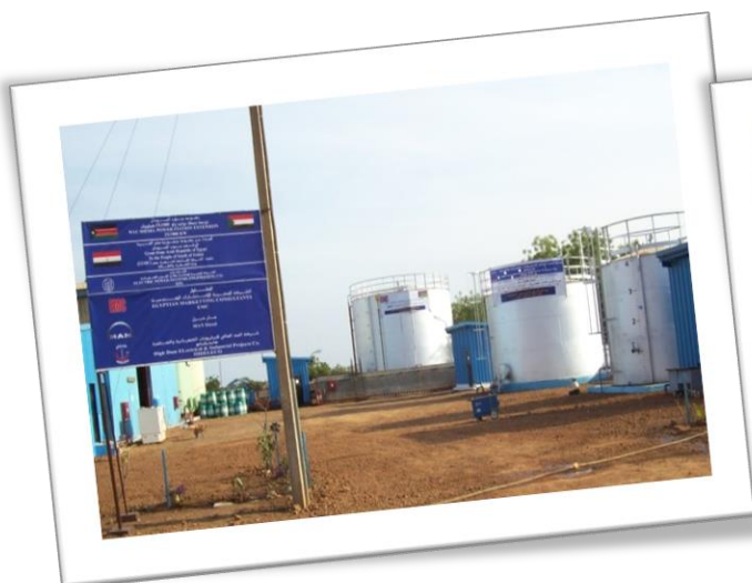
Wau Power plant over View
