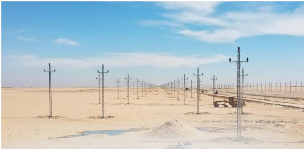
OverHead Transmission Lines 22kV
