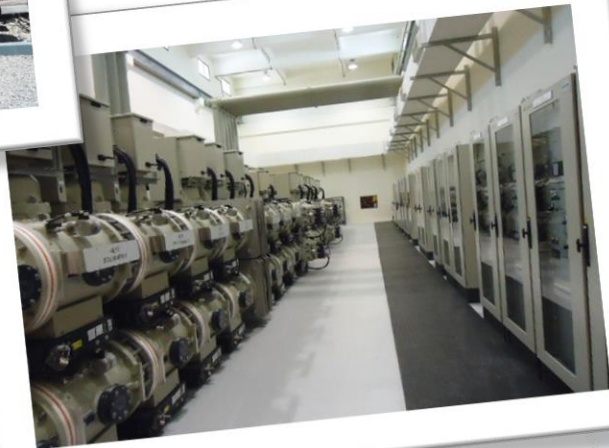
Main AC/DC Relay Sub AC/DC
