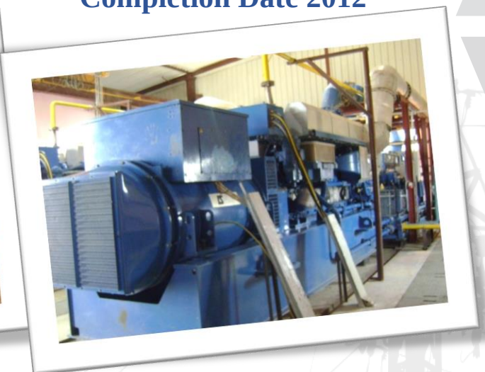
Diesel engines inside engine hall
