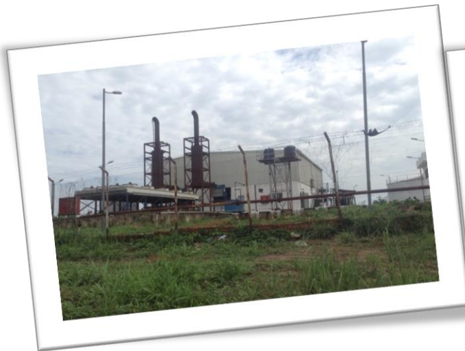
Yambio Power plant over View
