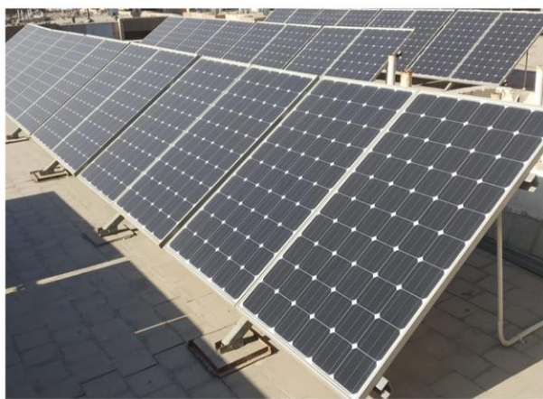
PV Solar power stations
