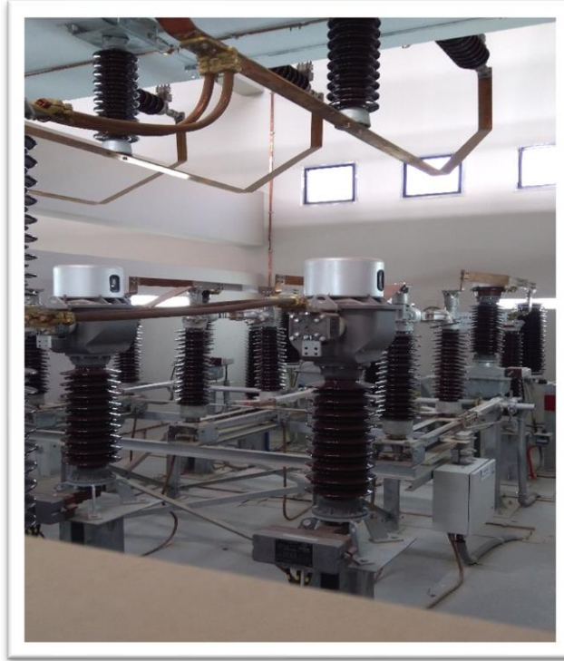
Conventional Indoor 66 kV Equipment
