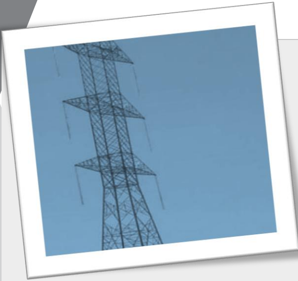
500 kV Double Circuit Tower
