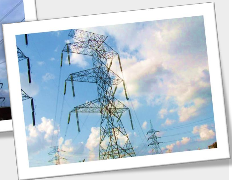
Multi Circuits Towers Approach to El-Siouf Substation
