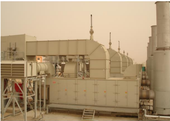
Karama Power Plant
